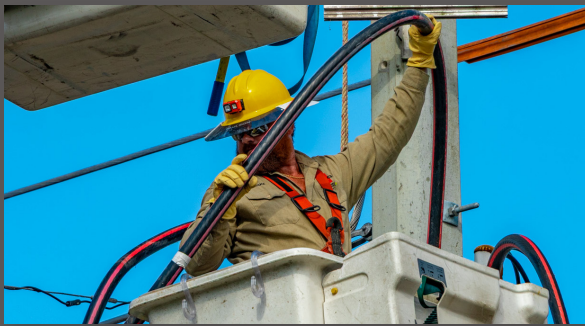
CHELCO Line Technician Jake Fain works on system hardening upgrades in Mossy Head.
